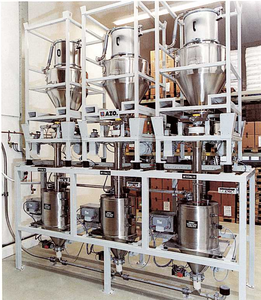
Feeding station for pneumatically filled AZO DOSITAINER®
