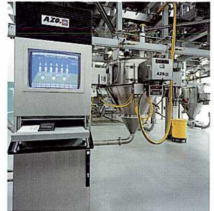
Control panel with color monitor
