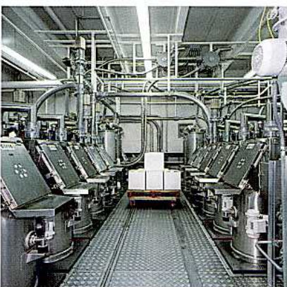
Discharging containers into the feed hopper
